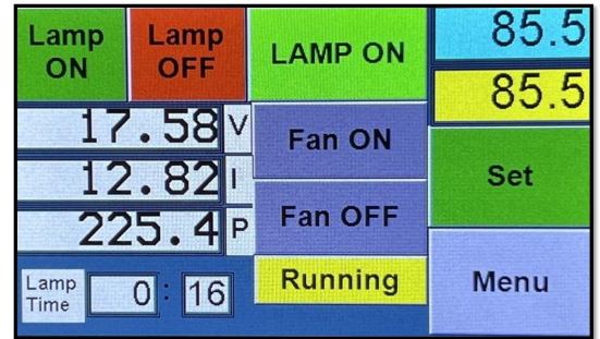
(Above) Touchscreen power supply main control screen
